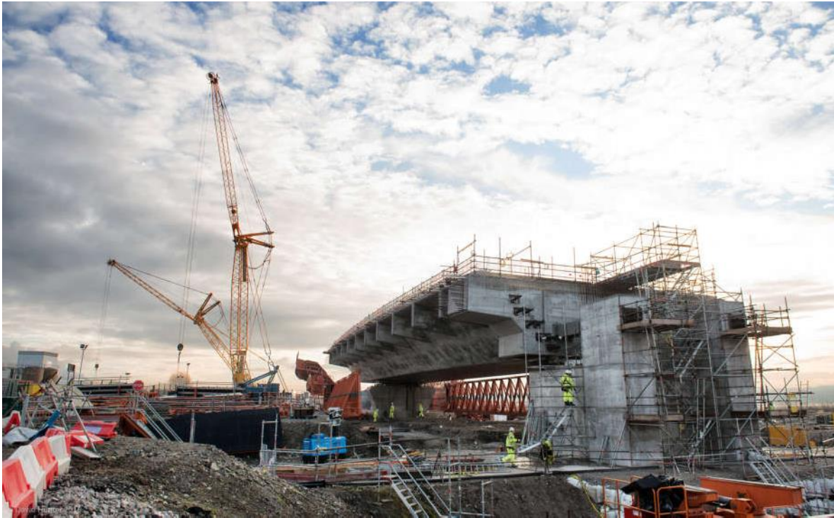
The first deck span of the Mersey Gateway's north approach viaduct showing the north abutment. (David Hunter).
