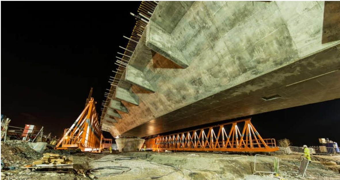
A close up view of the first concrete deck span for the Mersey Gateway's north approach viaduct. (David Hunter).
